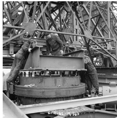
PS-08 vridbord installeras
